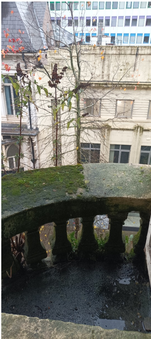
Buddleia growing from the Westgate's chimney stacks that will lead to the failure of the masonry ultimately and associated risk of falling masonry into the public realm.
