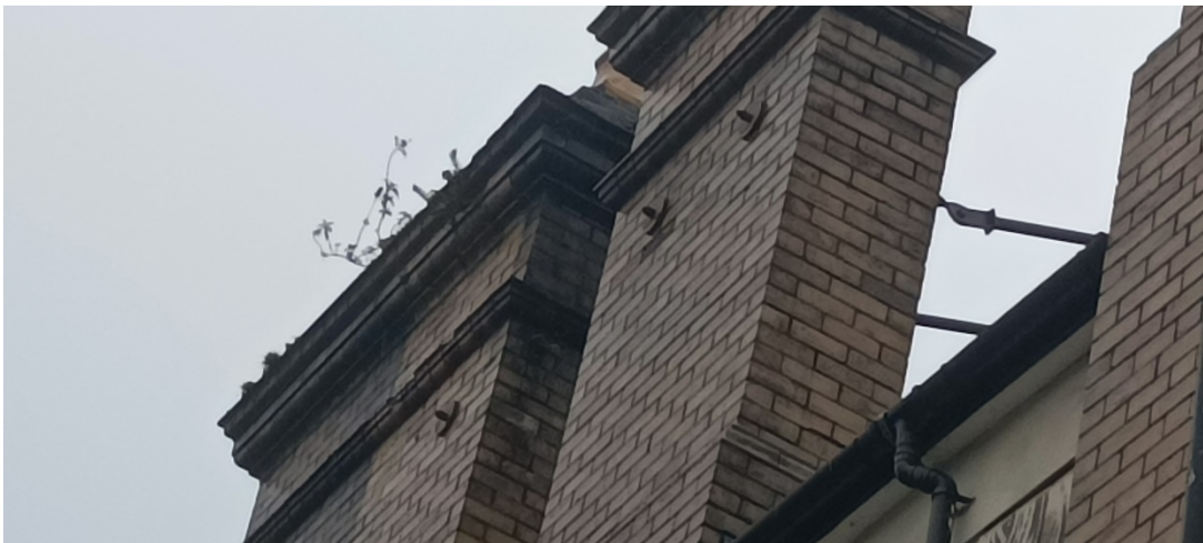
The lack of regular repointing and the failure of the cement render to the rear has permitted considerable water ingress. This will necessitate the removal of all cement render/removal of failed render and its reinstating with a lime render to allow for the drying out of the building's fabric.
