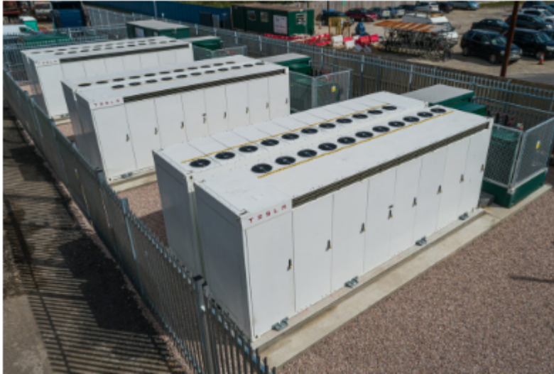
Taken from Power Systems UK website as an example of how such systems may look
