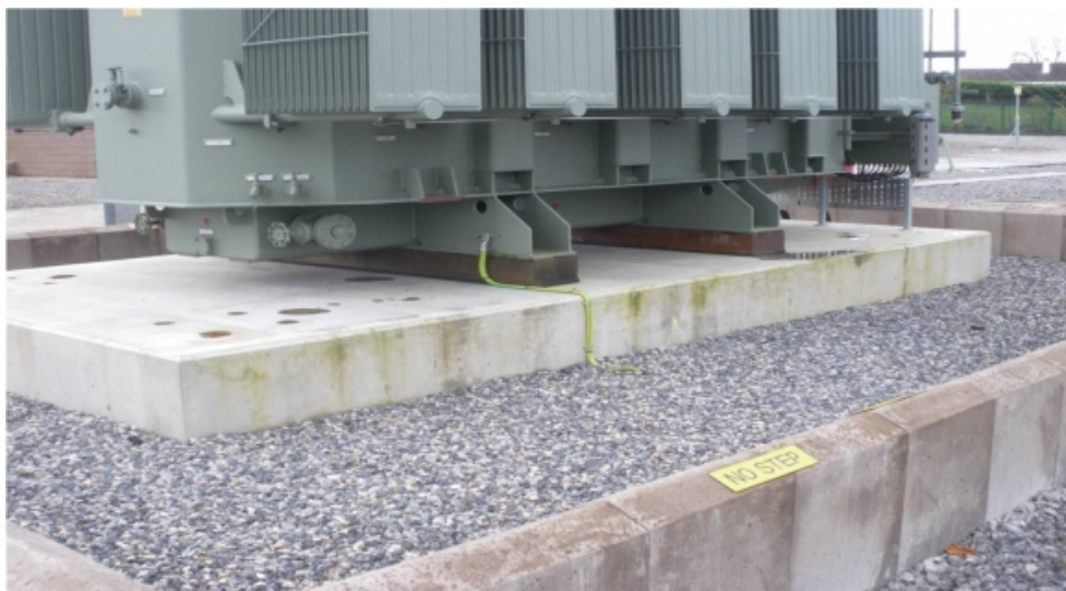
Example image of raised slabs or piers used for electrical infrastructure
